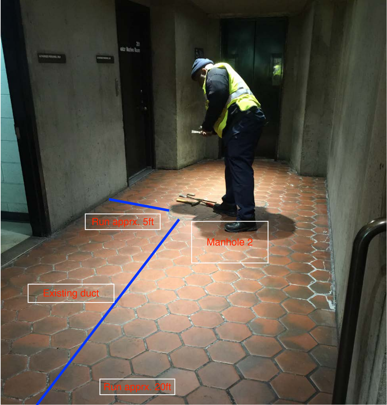
Picture 3: K01 Court House – Duct run from manhole 2 to AFC Panel
